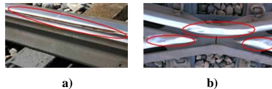
Fig. 1. Examples of damage to switch components: (a) part of the switch rail is detached and (b) damage due to plastic deformation and wear on crossing noses and wing rail [1]
